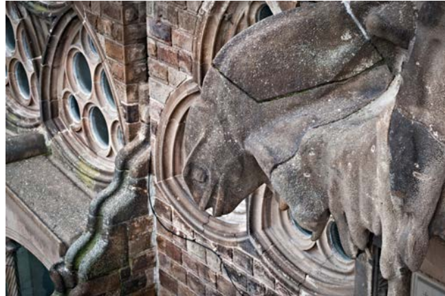
Gargoyle and windows in the cloister on the Nativity façade, in sandstone from Barcelona's Montjuïc mountain.
