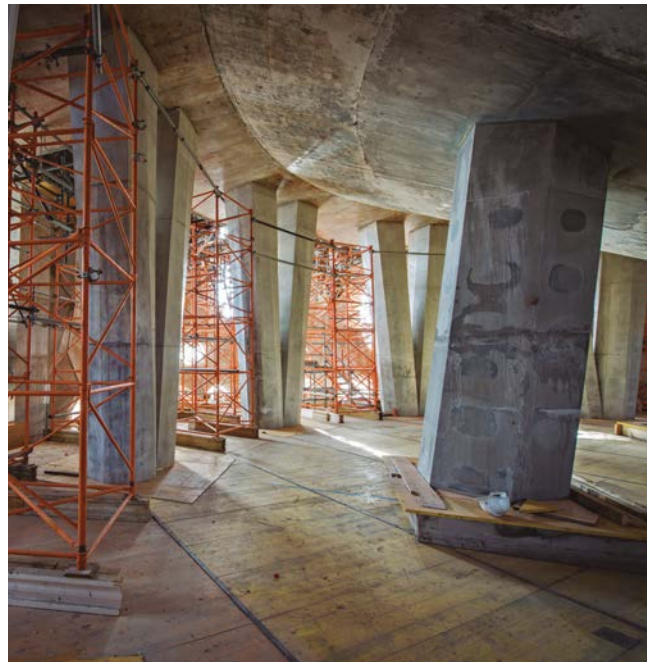
The support columns for the tower of Jesus Christ, as they pass through the lower part of the Crossing Room. They are exposed concrete.
