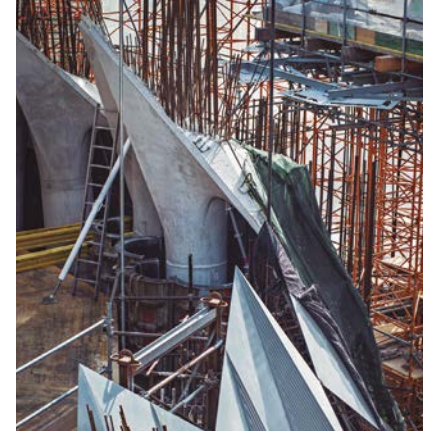
Columns and capitals in white concrete in the Crossing Room. The columns were poured on site using polyester moulds, and the columns were prefabricated using polyester moulds on the Temple grounds and then lifted into place with a crane.
